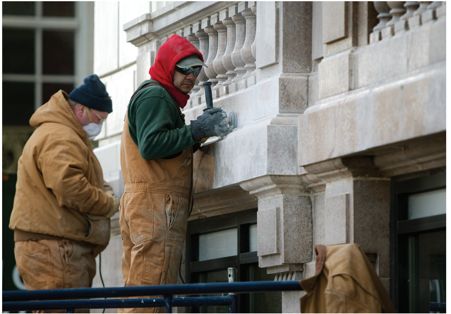
Workers repair the exterior of The Blackstone Hotel, 636 S. Michigan Ave., on Feb 19. The historic hotel is reopening after being closed for several years.
