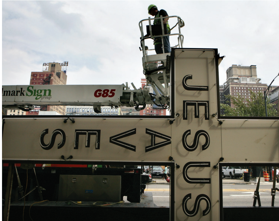
Construction workers take down the Pacific Garden Mission's signs on Sept. 25. The mission is moving to 1458 S. Canal St.
