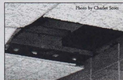
The capital improvement plan is designed to repair problems like this ceiling at South Side College Prep.
