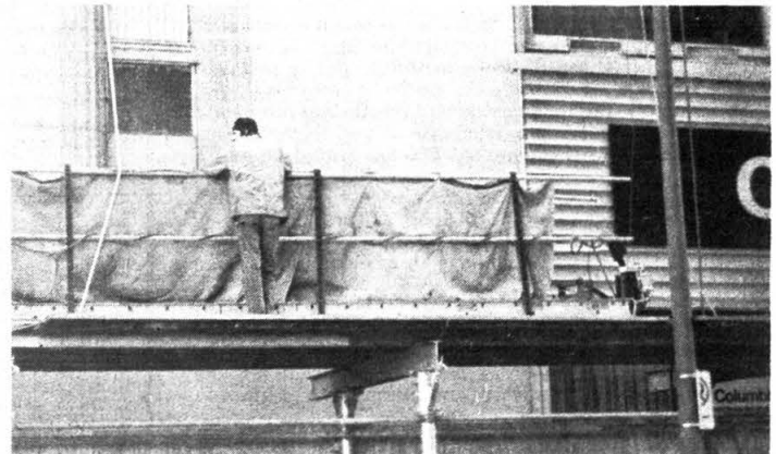
Work continues on the exterior of the Michigan campus (Photo courtesy of Daphne Young) See Joseph Collins' story on opposite page.
